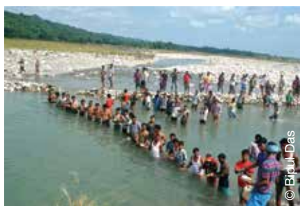
Step 2: Construction of Dong Bundhs before the onset of the dry season (Dec-April).
