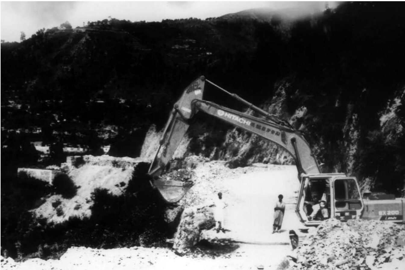
Infrastructure development in Abbottabad has been allowed to proceed without recourse to environmental impact assessments or land use zoning.
