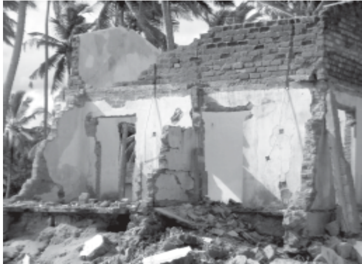
Damaged dwelling near Nilwella; Bhagya Gunasekera © IUCN
