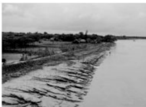
Riverbank erosion in Noakhali. PHOTO: Ahana Adrika
