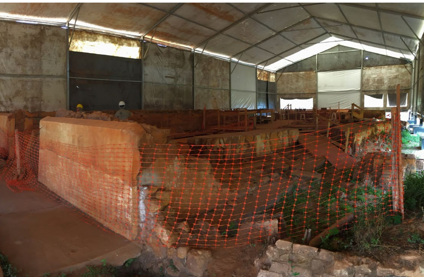
Above: Rio Doce Panel and Renova Foundation technicians visit the interior of the church impacted by the mud. Paracatu de Baixo, district of Mariana, Minas Gerais. September 2017. Photo: IUCN/Rio Doce Panel archive
