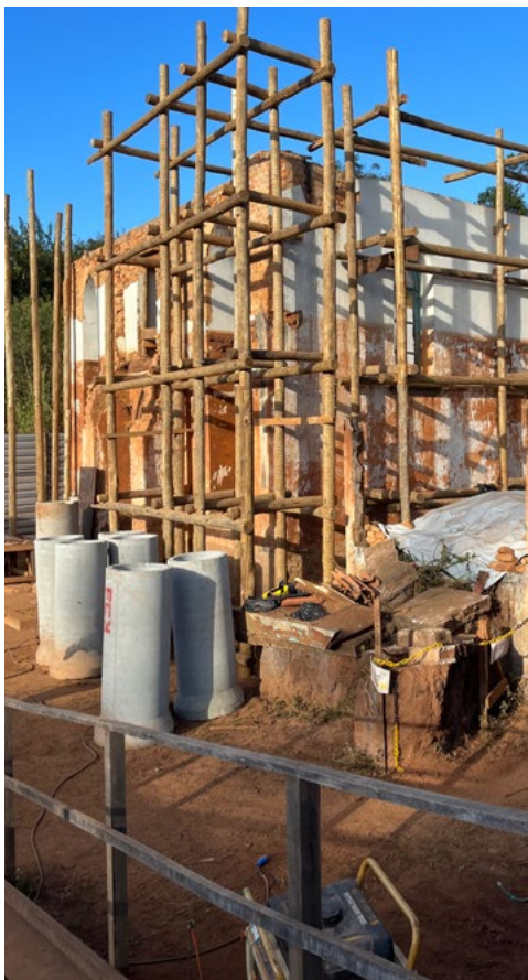
Above: Restoration work on the church affected by mud in Paracatu de Baixo, Minas Gerais. July 2022. Photo: IUCN/Rio Doce Panel archive
