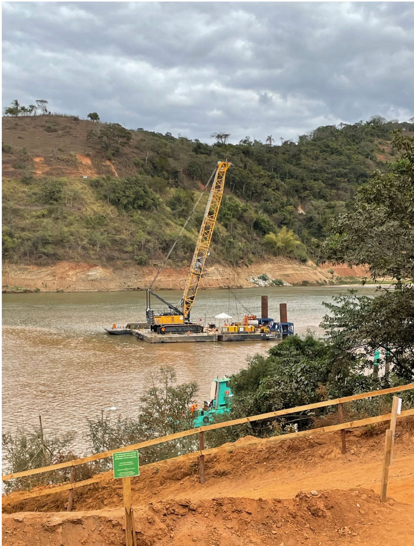
Above: Works on the reservoir of Risoleta Neves Hydroelectric Plant (Candonga). July 2022. Photo: IUCN/Rio Doce Panel archive
