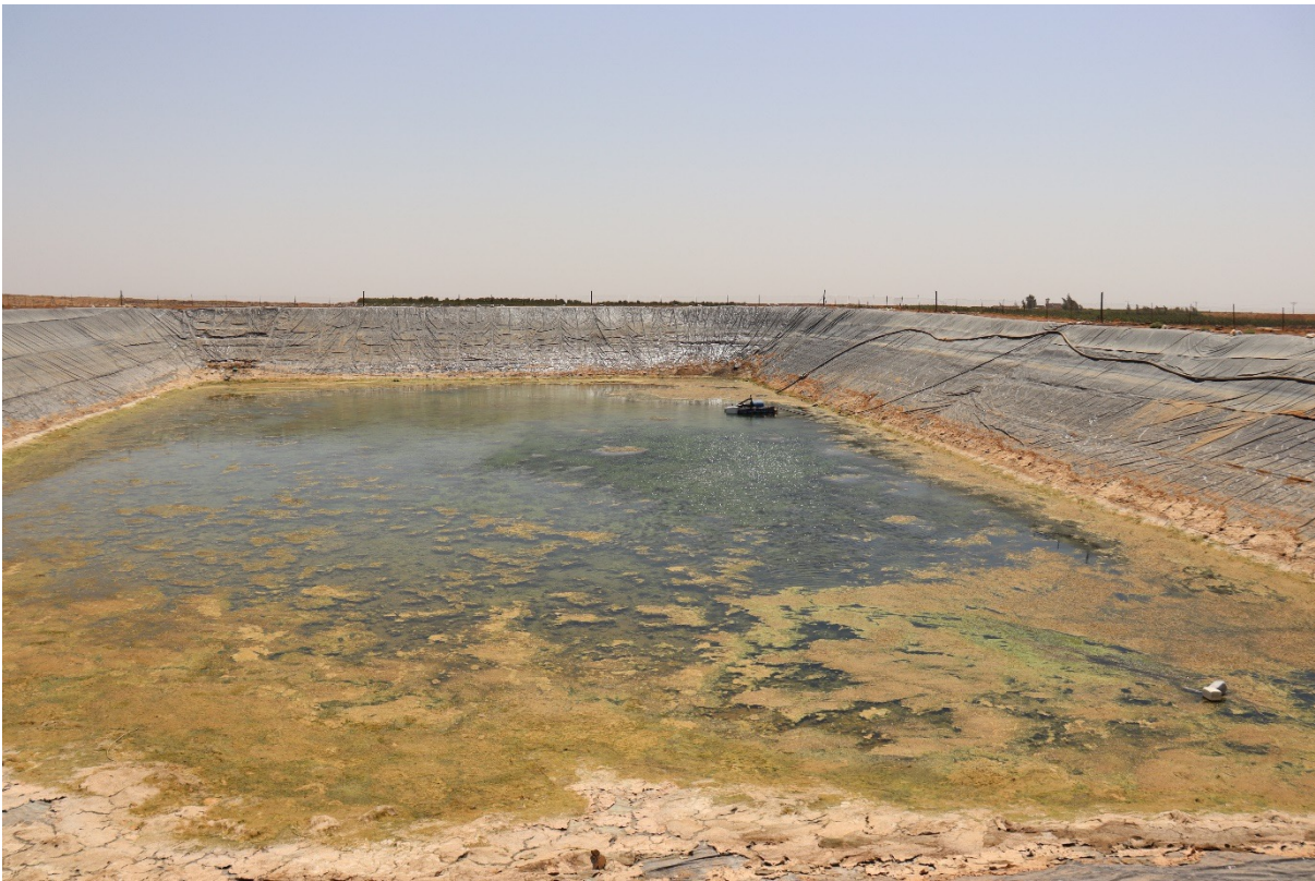
Figure 7: Deteriorated plastic lining in water ponds that are used for irrigation water storage
