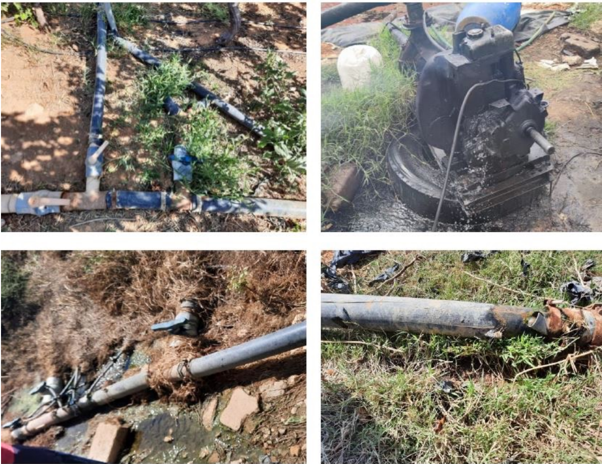
Figure 6: Observations from the evaluated farmlands indicating deterioration of irrigation system components
