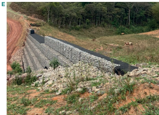
Sediment-retaining dike built to mitigate the impact caused by top-mountain erosion (visible on the top left corner of the photo) in local water courses
